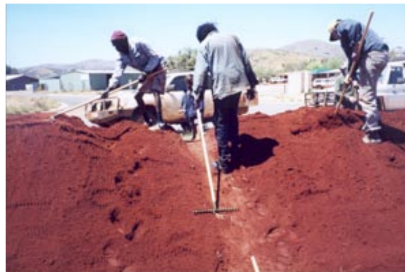
2. View of enthusiastic workers shaping the first mound at Pipalyatjara. The top is flattened off and the general shape of the profile is being formed [October 2000].
