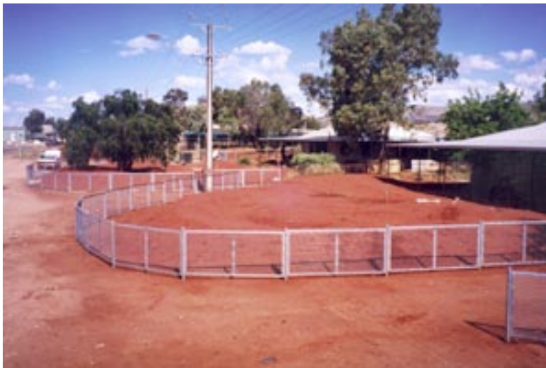
23. View of a finished mound system in a front yard at Pipalyatjara surrounded by the newly designed pannel fence. The mound in the back ground surrounding two peppercorn trees was the first to be built in a front yard
