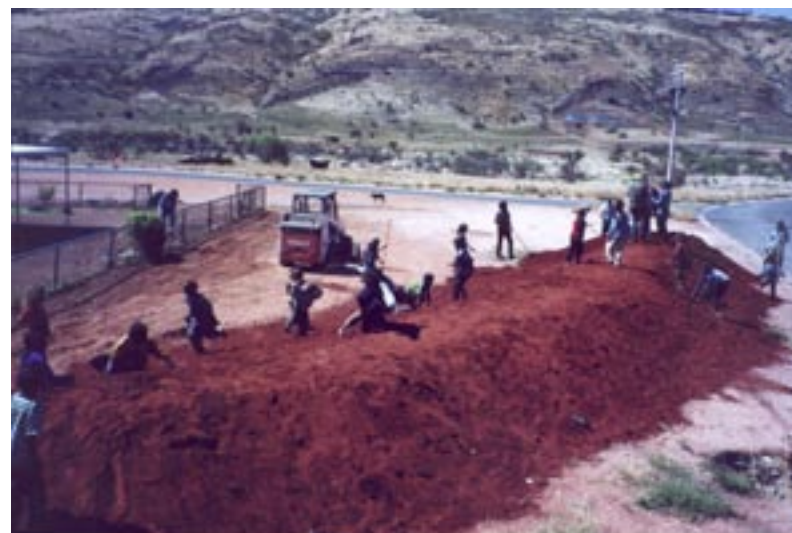
4. View of the first half of the crescent shaped mound being built to fill the median strip at Pipalyatjara. Note the flat top on the mound for sitting and standing [October 2000].
