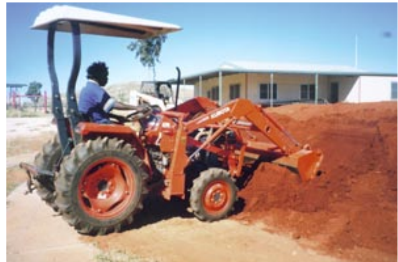
16. A small tractor with a front end bucket was effectively used to drag soil out from the Amphitheatre and produce a gradual side slope [May 2001].
