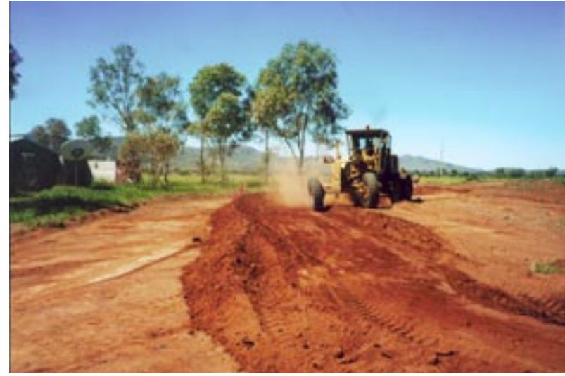
6. This ponding bank was designed to collect and drain storm water from the main internal road system to an open area outside the community [March 2001].
