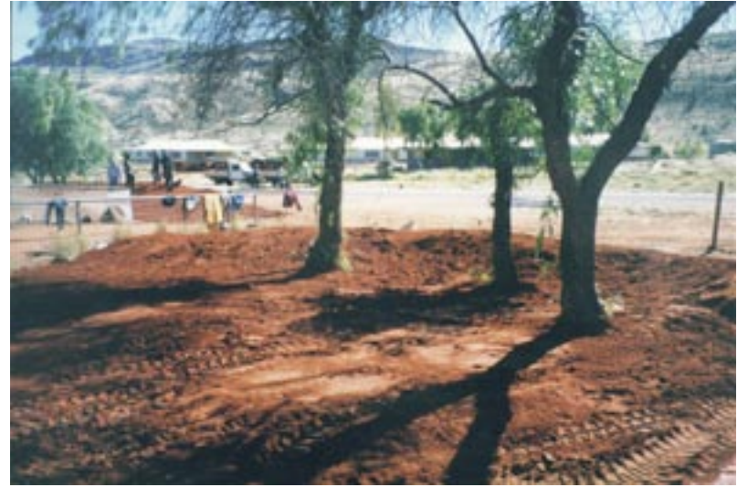
6. Mounds like this one were built in open areas around the community to collect storm water, thus preventing it from draining into the road system [May 2001].
